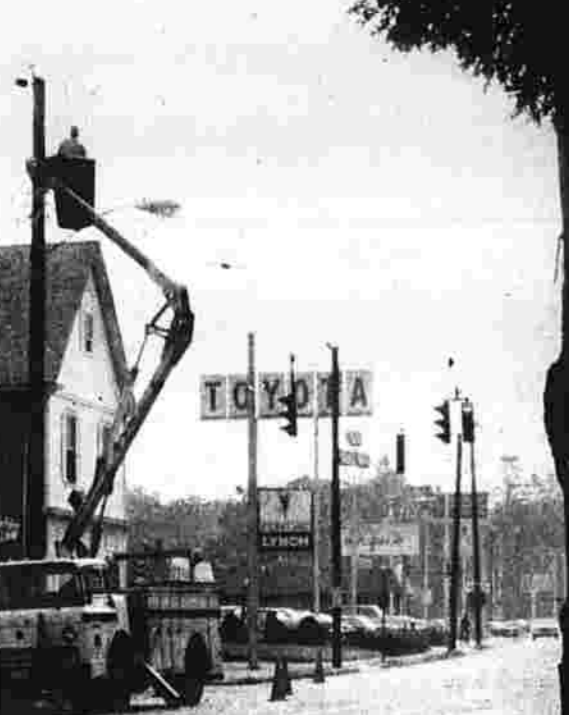
Workers repair traffic signals at the intersection of Center and West Center Streets this morning which were damaged during last night's thunderstorm.
